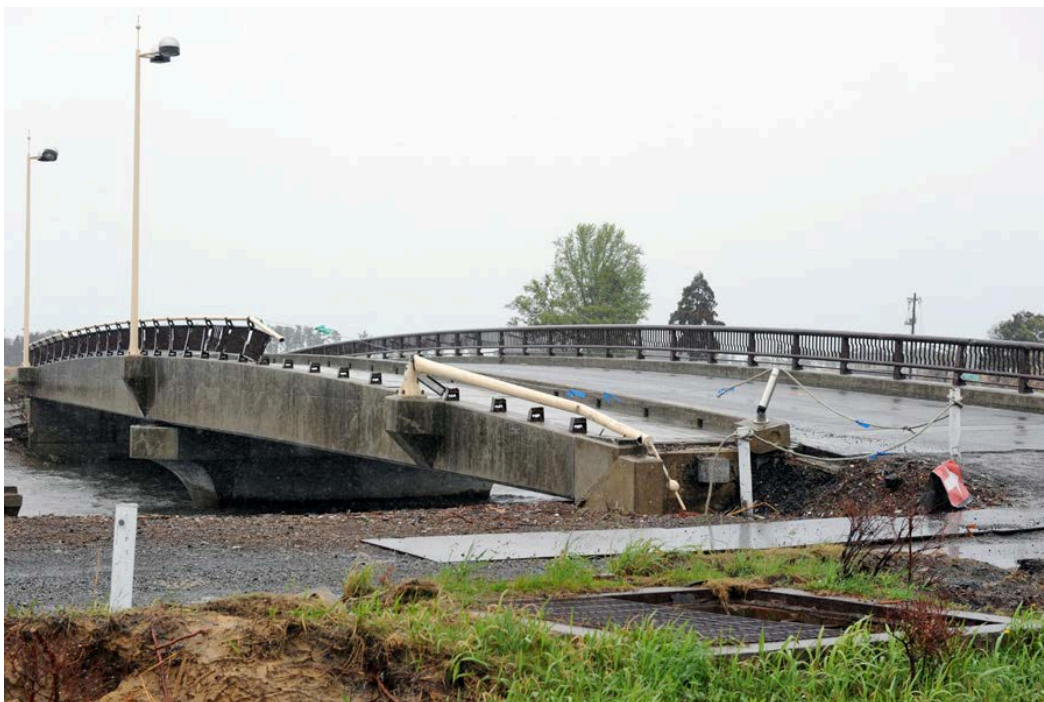
Figure 9 Bridge in Japan with minor-moderate damage of the superstructure and some minor scouring in the foreground. Source: Structural Engineers Association of Washington.
