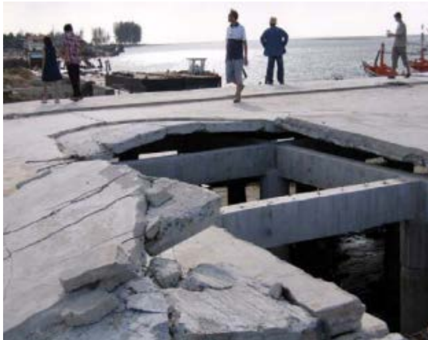
Figure 20 Damage to a wharf deck in Thailand from vertical buoyancy forces. Source: PARI, 2009.
