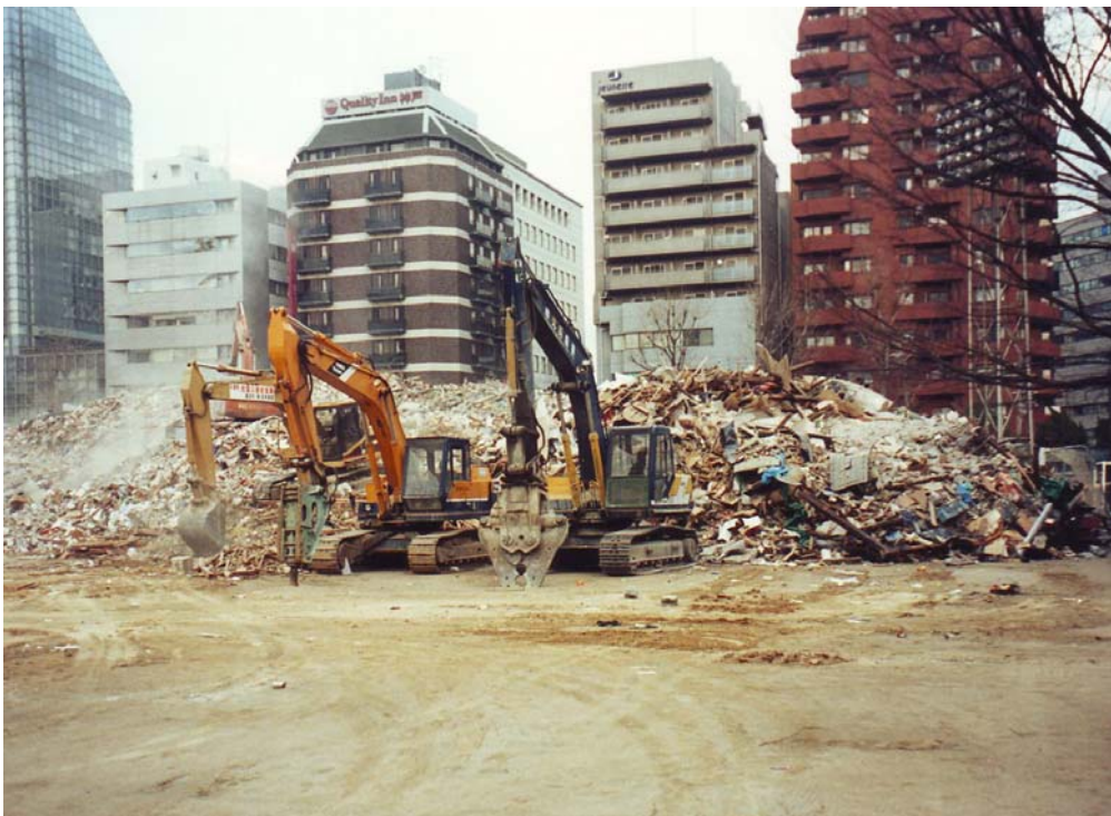
Figure 1 Rubble from collapsed buildings being stockpiled on a soccer field, Kobe 1995 (photo Jim Cousins).
