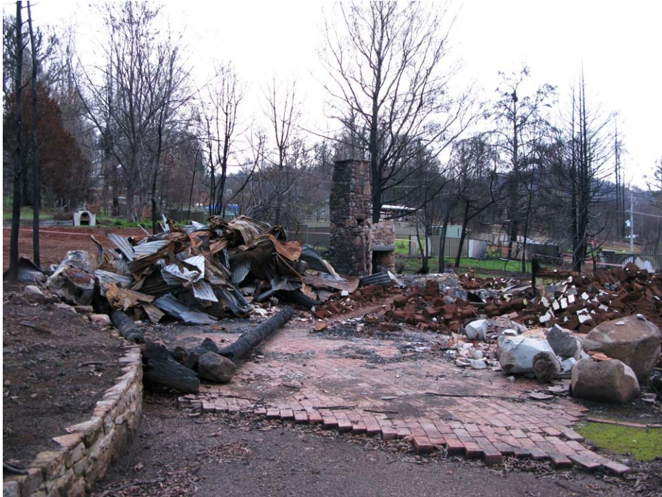
Figure 4 A typical house-lot mid-demolition following the devastating Victorian Bushfires (Australia) February 2009. The intense heat and destructive capacity of the fires led to over 3000 homes requiring demolition and debris disposal. Due to the scale of the event, the Australian government elected to let a single contract for all demolition and debris disposal at existing landfills and some incidental recycling (photo Charlotte Brown).
