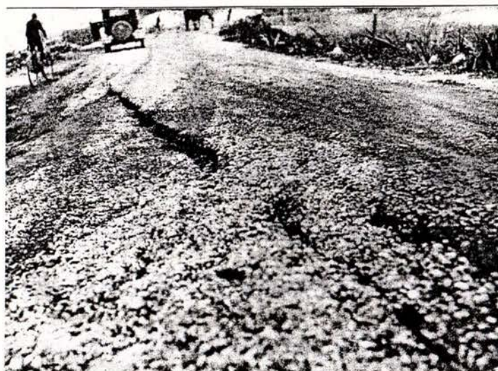
Figure 3-21. Cracks in Preston Road at Blaketown ( New Zealand Free Lance , 26 June 1929)
