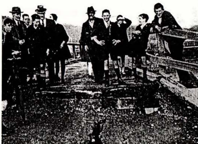
Figure 3-20. Blaketown Footbridge- note the settlement of the approach embankment ( Auckland Weekly News , 3 July 1929)
