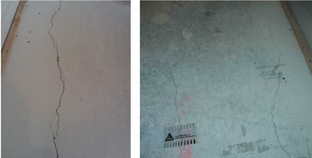
Figure 2. Pacific tower floor cracks after Christchurch earthquake 2011
